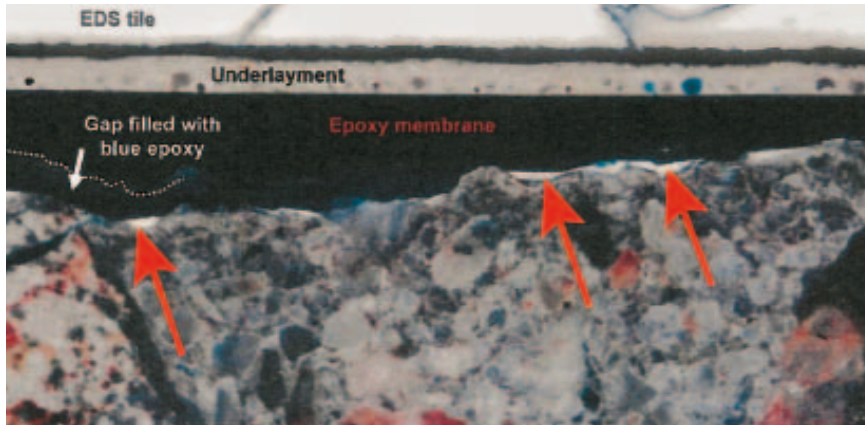
The layers of the floor system with arrows pointing to the white areas (silica gels) on the surface of the concrete.
