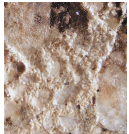
The surface of the lab sample shows lithium silicate applied to the sand-blasted concrete surface.
